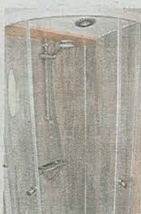
The large quadrant shower cubicle.
