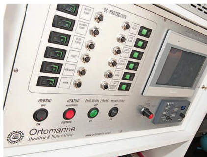
Touch screen displays boat's electrical systems
